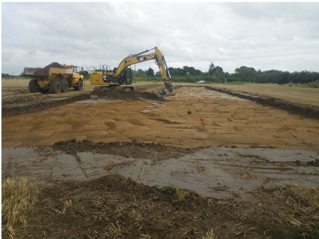
Plate 2 – Working shot showing topsoil stripping revealing the underlying clayey sand natural substrate, 13001, looking east
